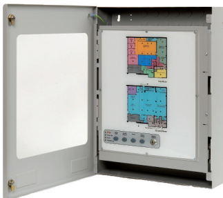
View showing mimic mounted on inner door
